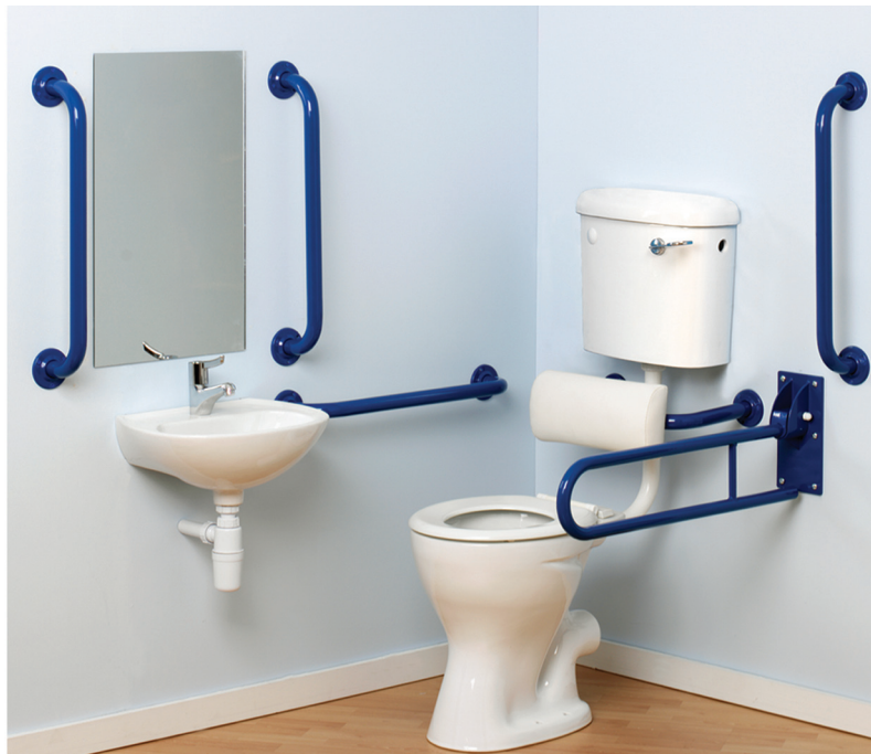
Figure 3: Toilet that complies to Part M of building regulations
